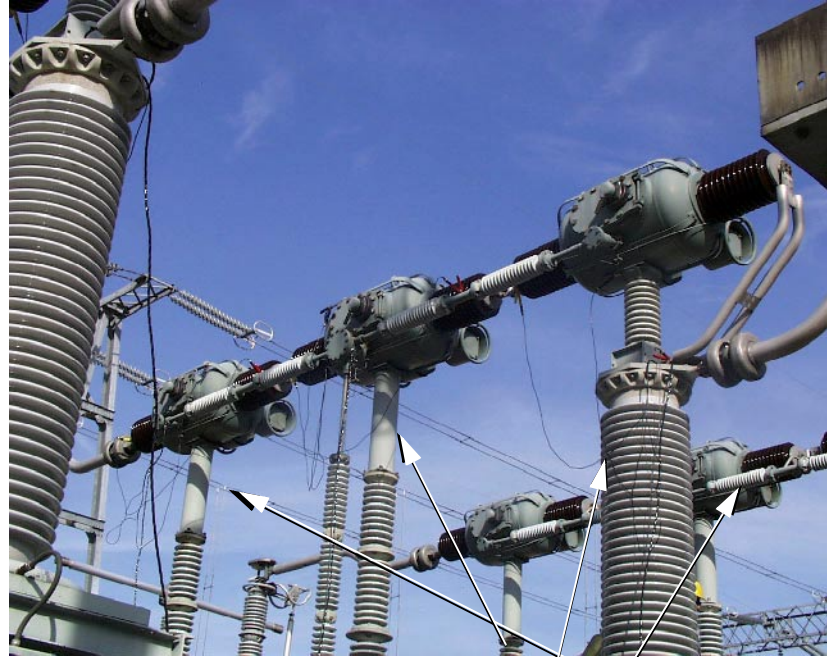
EHV Contact Monitor Cabling
